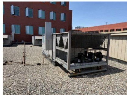
Pic #2 another view of existing YORK/Fisen RTU
