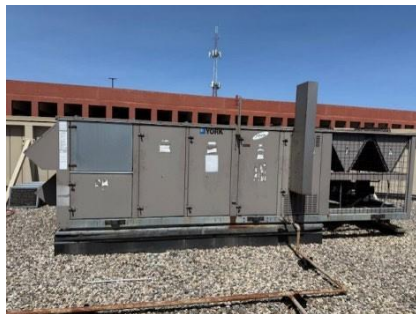
Pic #1 existing YORK/Fisen RTU
